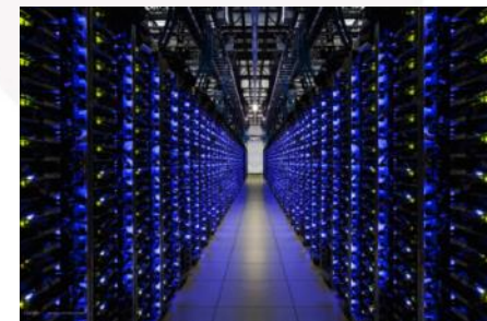
Data centres and e-infrastructures
